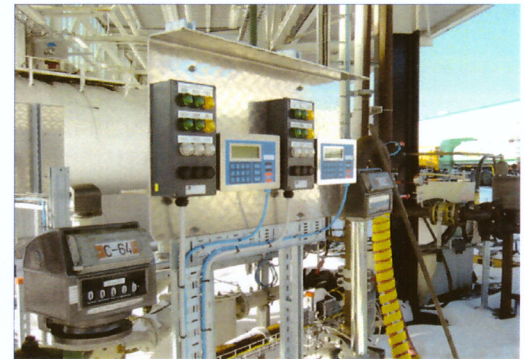
A typical installation at a truck loading facility with indicator panels, MFT1000 display units and traditional flow meters.
